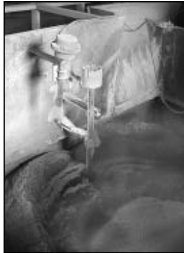
A concrete manufacturing plant has installed a new Model KA unit in the pictured bin. This bin is filled with stone, but Model KAs are also being used in this facility with steamed sand, gravel and cement.
